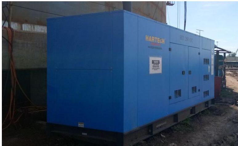
GENERATOR SET (FOR SITE JOB)
